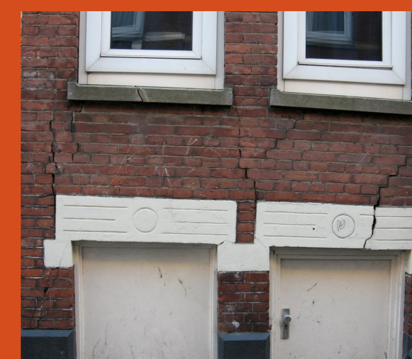
Functional damage: the functionality of doors, windows and underground service lines are affected.
