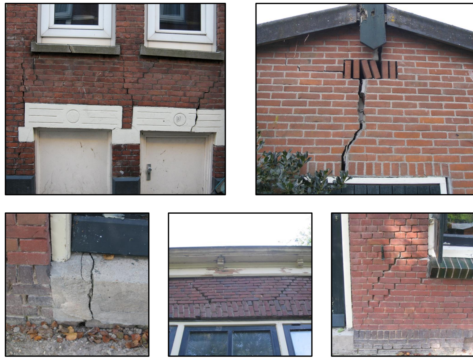
Figure 1. Examples of cracking damage to buildings due to settlements.
